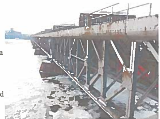
L & D 15 Service Bridge
