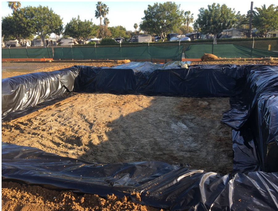
BMP Implemented – Sediment Trap
