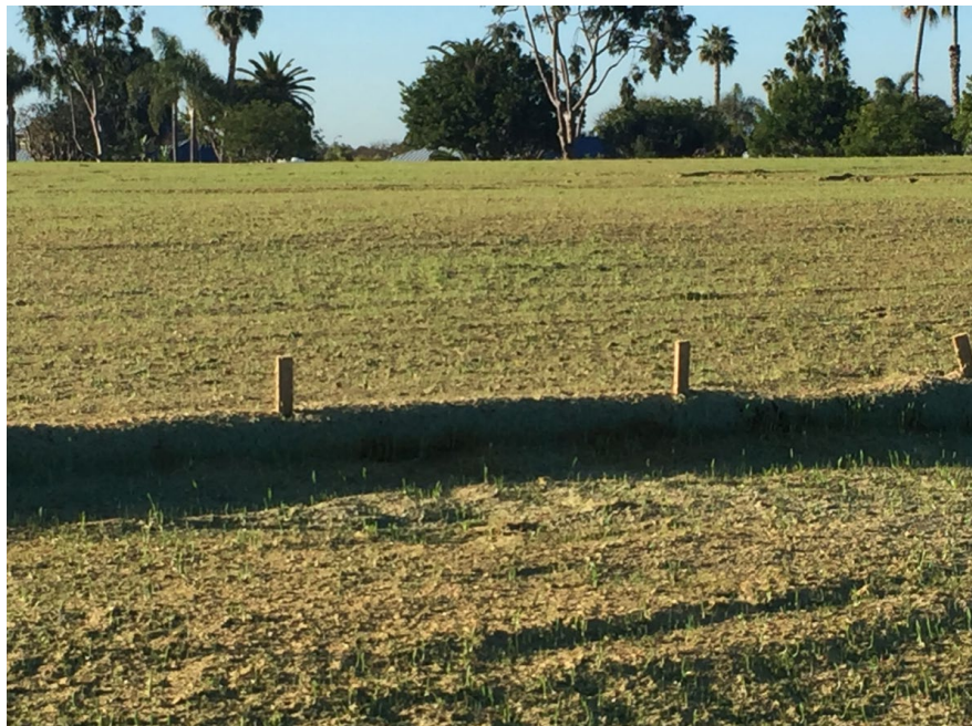
BMP Implemented – Fiber Rolls and Bonded Fiber Mulch with Hydroseed one week after installation
