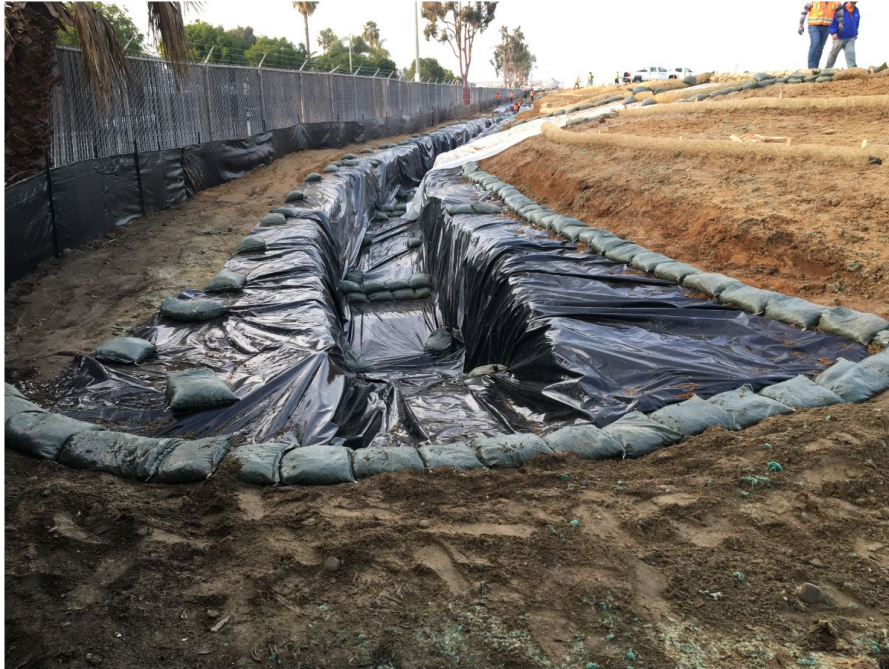
BMP Implemented – Sediment Trap
